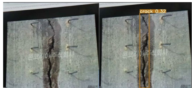
a) Original image b) Crack detection image
