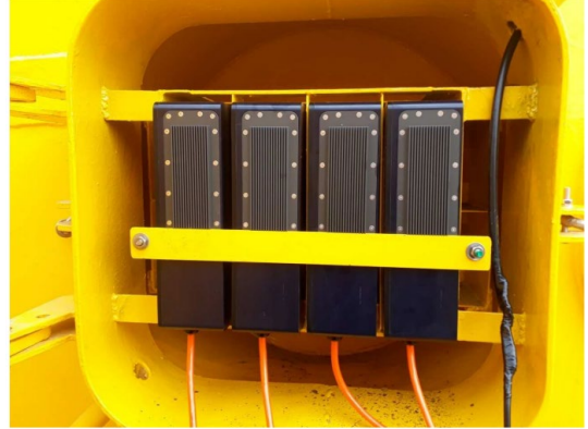
Fig. 5. Four seawater-based marine specialized batteries for light buoy
